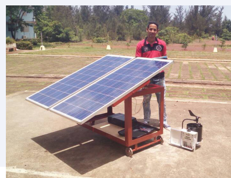
Photovoltaic mobile module at ISMMM.
