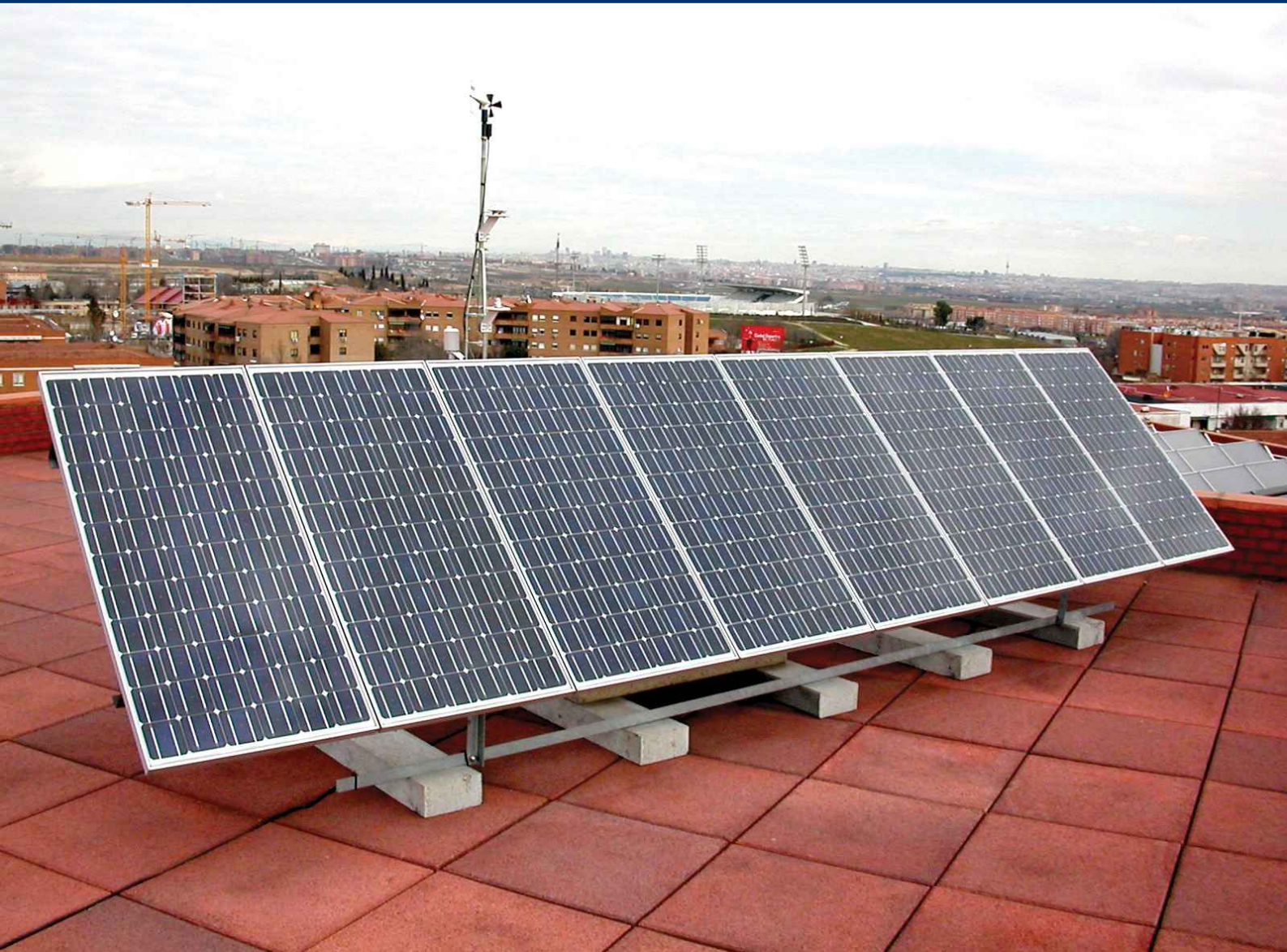
Photovoltaic experimental installation of the Power Control Group.
