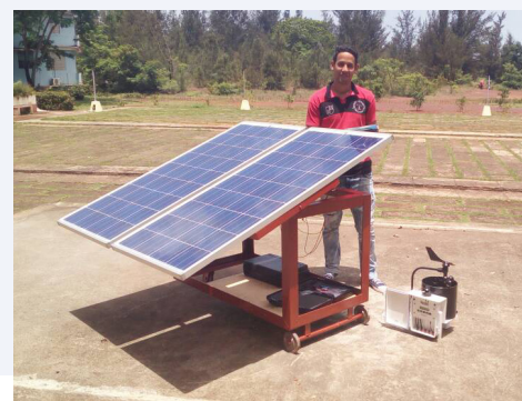
Photovoltaic mobile module at ISMMM.
